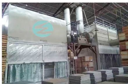
干磨机除尘 Dry squaring machine dust removal
