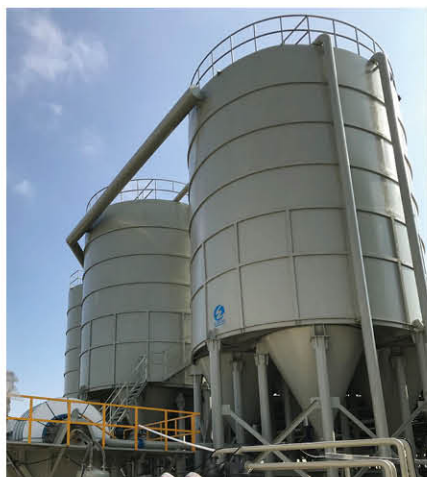
肇庆将军陶瓷污水处理系统 Zhaoqing General Ceramics Sewage Treatment System
