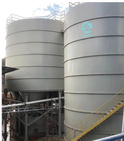
广西新瑞福陶瓷污水处理系统 Guangxi Xinrui fu Ceramics Sewage Treatment System
