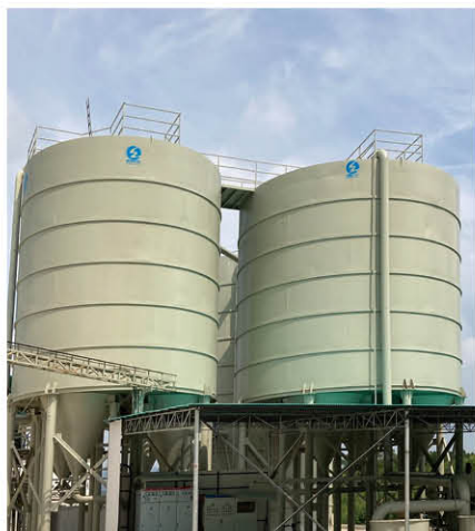
广东华陶建材污水处理系统 Guangdong Huatao Building Materials Sewage Treatment System
