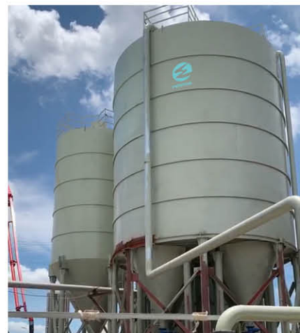
肇庆宏润陶瓷污水处理系统 Zhaoqing Hongrun Ceramics Sewage Treatment System
