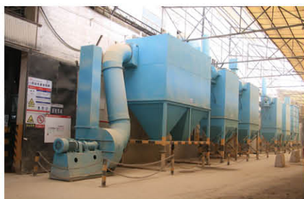
压机除尘 Press dust removal
